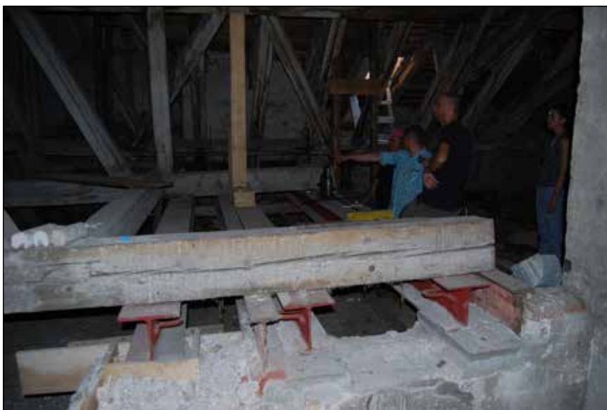
■ Foto 6. Intervenții de consolidare a șarpantei istorice © Bogdan DEMETRESCU ■ Photo 6. Consolidation interventions on the historic roof structure © Bogdan DEMETRESCU
