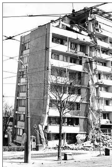
■ Foto 6. Blocul Lizeanu, colaps parter, 4 martie 1977 ■ Photo 6. Lizeanu Apartment Block, ground-floor collapse, March 4, 1977
